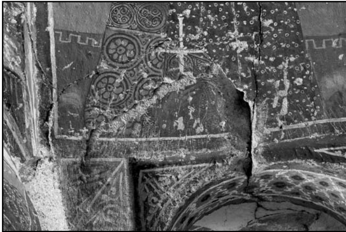
Fig. 7: Avcılar, church of Yusuf Koç, structural instability in walls
