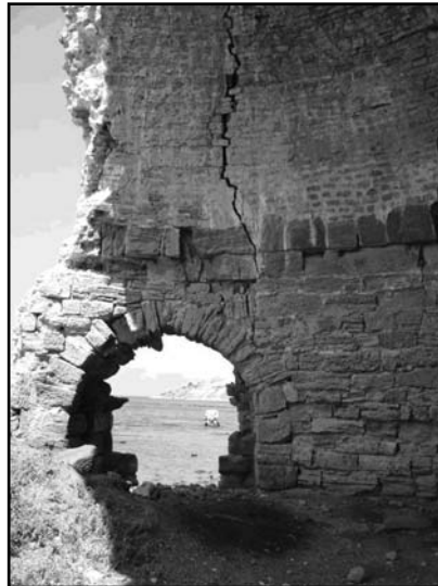
Fig. 4: View of West tower with crack in the dome
