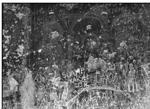
Fig. 12: Şahinefendi, church of Forty Martyrs of Sebaste, the pictorial surface covered by deposits of particled carbonaceous, of signs of vandalism, inscriptions and gaps
