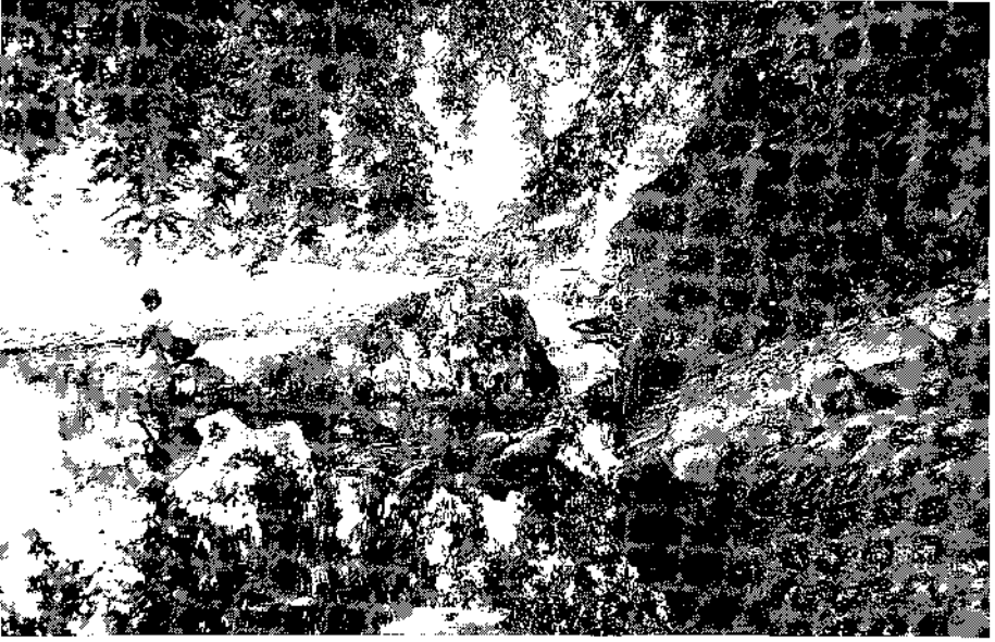
Illustration 15: Kaledran kiosk, Kaledran, collapsed segment of pavilion wall partially submerged in the Kaledran Çayı
